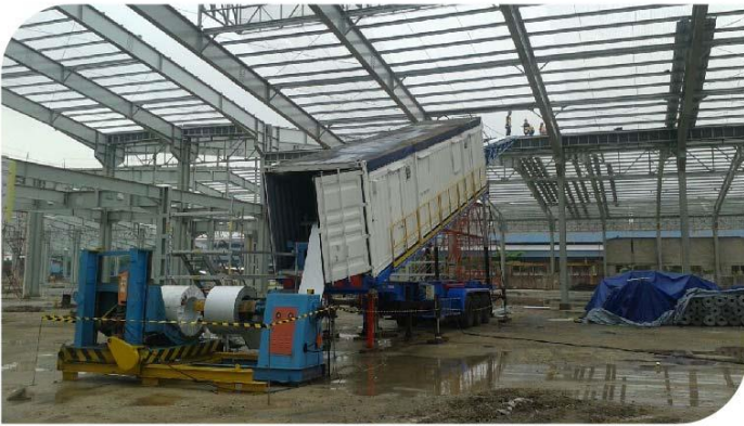
Mobile Elevated Rollforming (MERF) System
